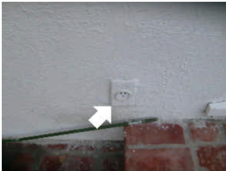
The exterior plug in the back patio and the switches at the pool equipment do not have the proper weather caps.
