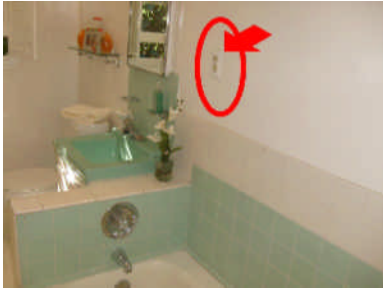
Not Acceptable. the outlet on the wall is close too the tub and is not GFCI protected for safety.
