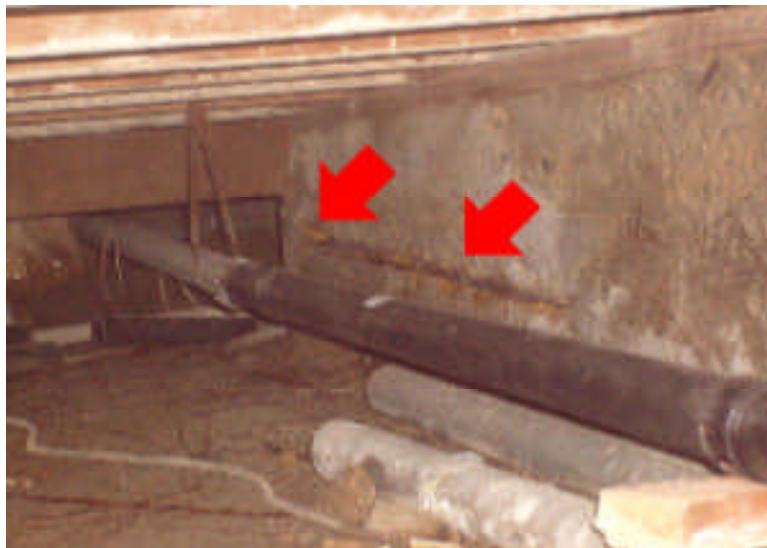
Rusting exposed rebars
