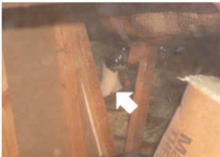
unencapsulated older insulation
