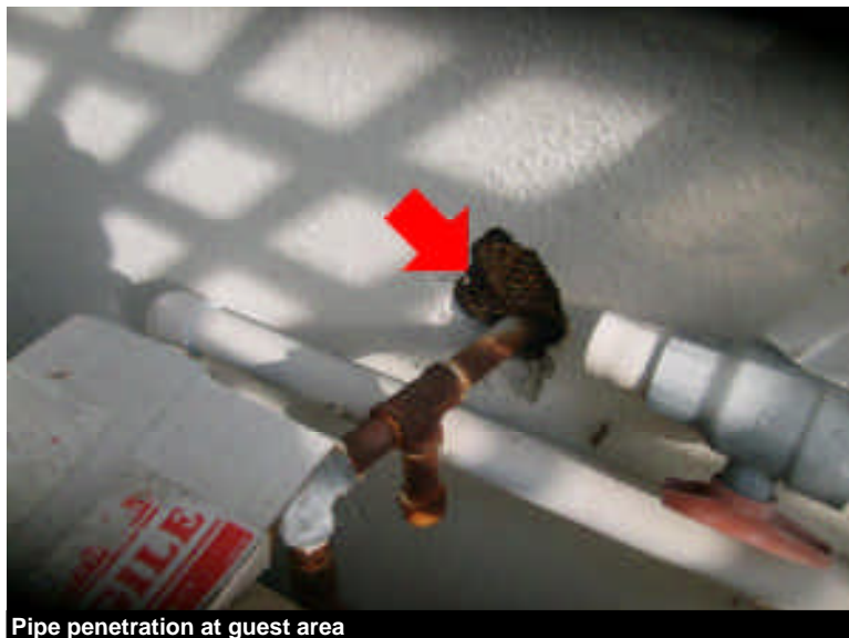
Pipe penetration at guest area
