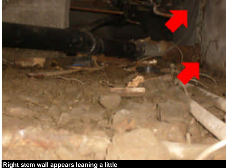
Right stem wall appears leaning a little This area of damp soil also is showing the stem walls leaning a little and the sloping floors in the front hall indicate some settlement has occurred.
