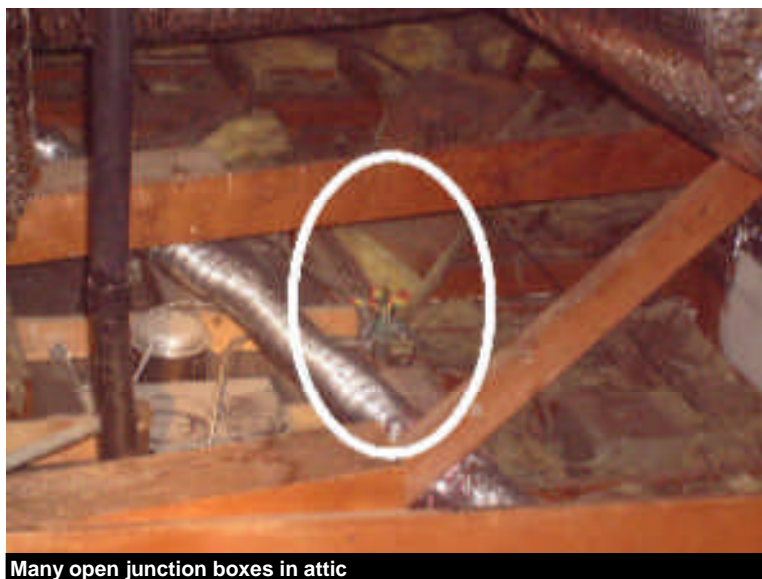
Many open junction boxes in attic
