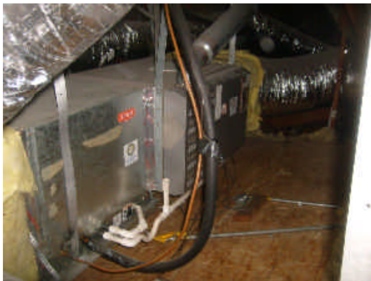
The heating unit is located inside the building in the attic.
