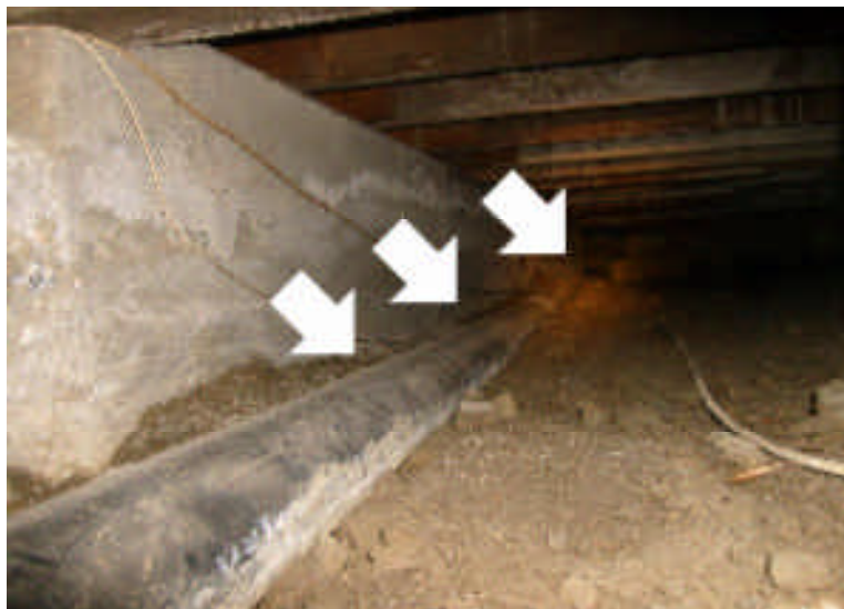
Laying on the ground, uneven, poor slope
