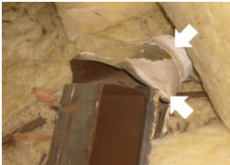
Loose old sections with insulation
