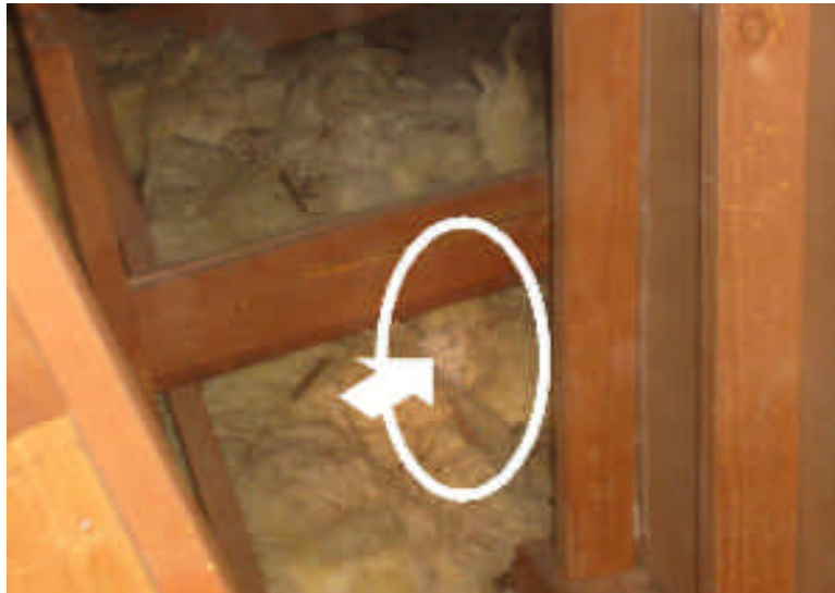
Loose piece of insualtion
