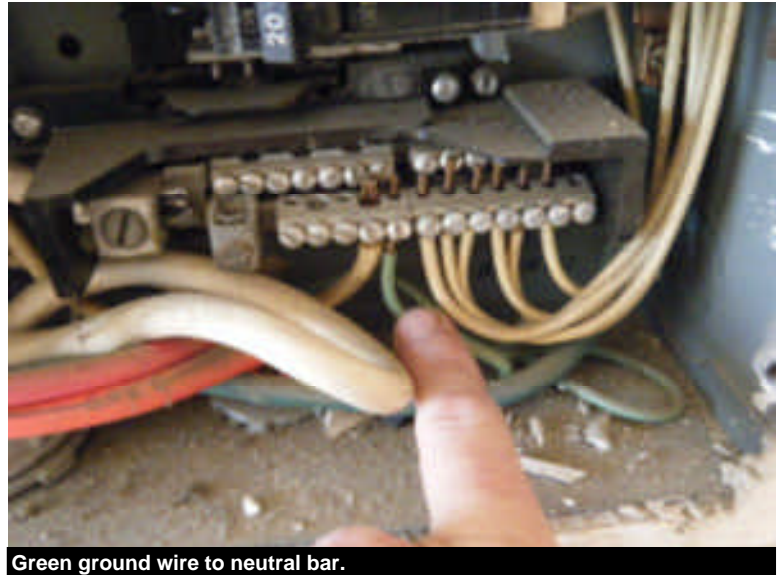
Green ground wire to neutral bar.
