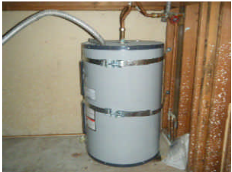
The water heater is located in the closet under the stairs.
