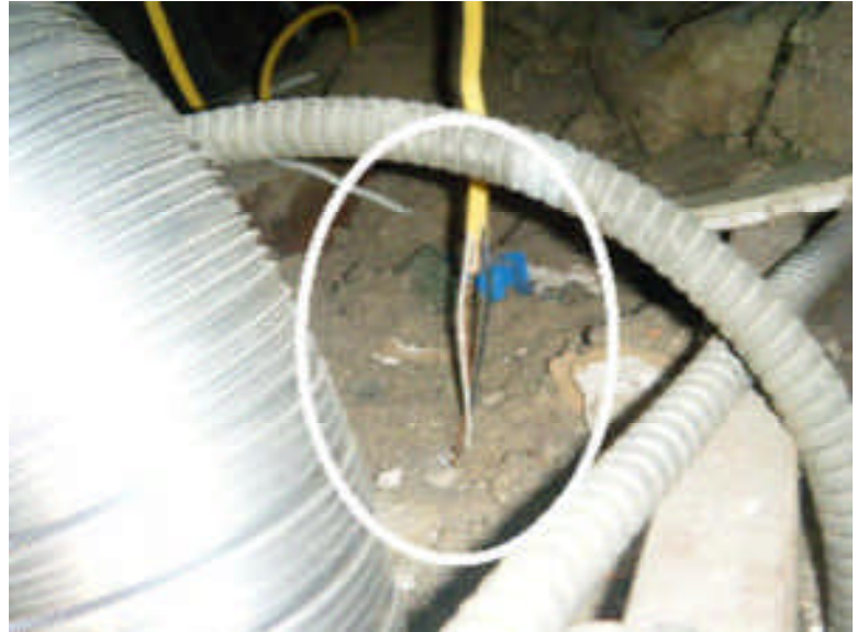
There are exposed wires in the attic with no wire nut caps and left in a unsafe condition.
