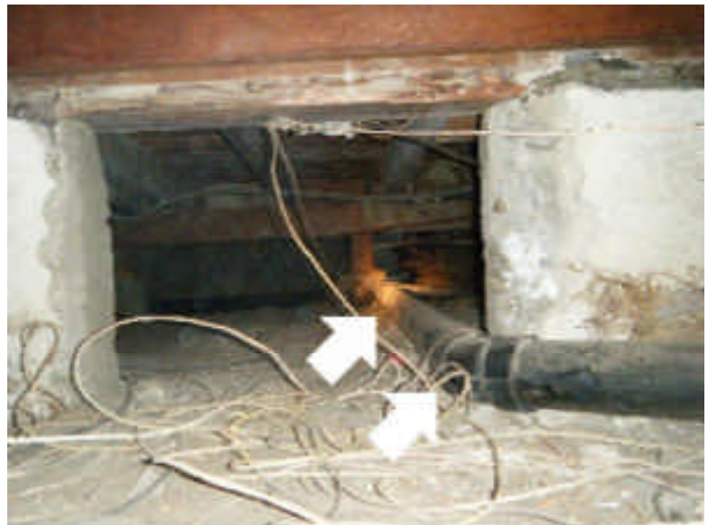
Needs Attention, The waste/drain lines have areas of incorrect slope as the line slopes down and then back up such as at the hall shower drain and there is a very flat area in the middle of the house. This may cause it to block up or fill with sediment and drain poorly and should be repaired by a plumbing specialist.
