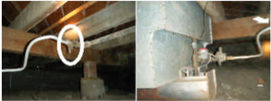
The gas is shut off to the furnace under the house.
