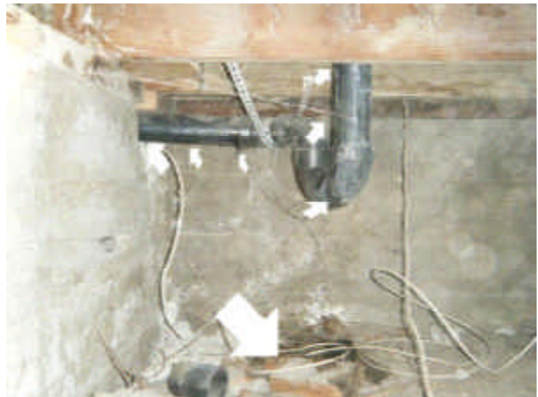
Leak under the hall shower also has the drain line go uphill a little as passes through the concrete stem wall.
