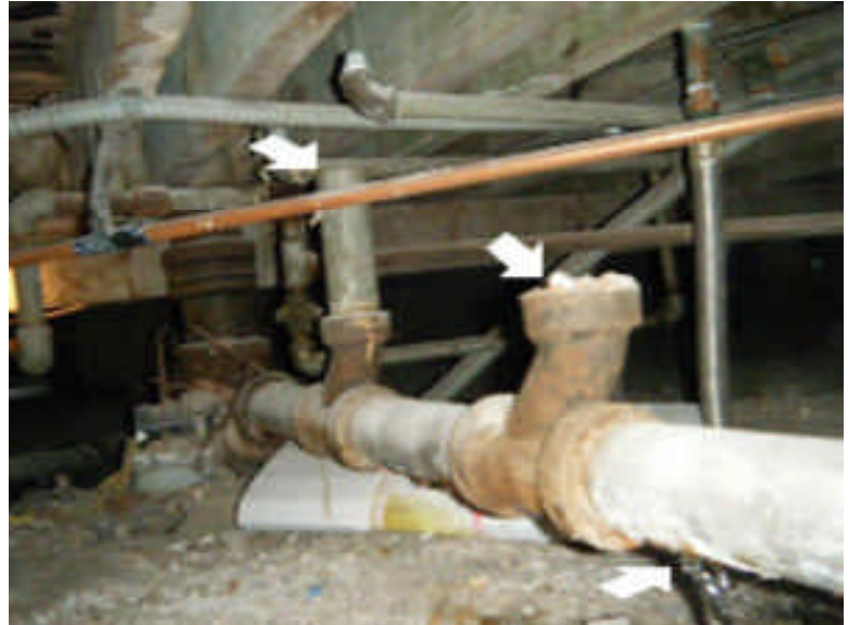
Kitchen drain area has old pipes , rusting and needing repair and some of the old pipes do not appear sealed or capped off properly.
