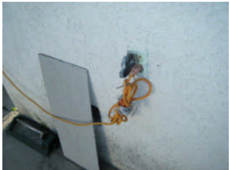
Needs Attention, there is an extension cord plugged in to the back outlet for an out side light. If this is continued to be used it should have a different rain guard type cover
