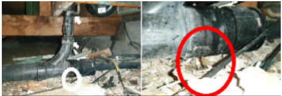
Master bath drain area
