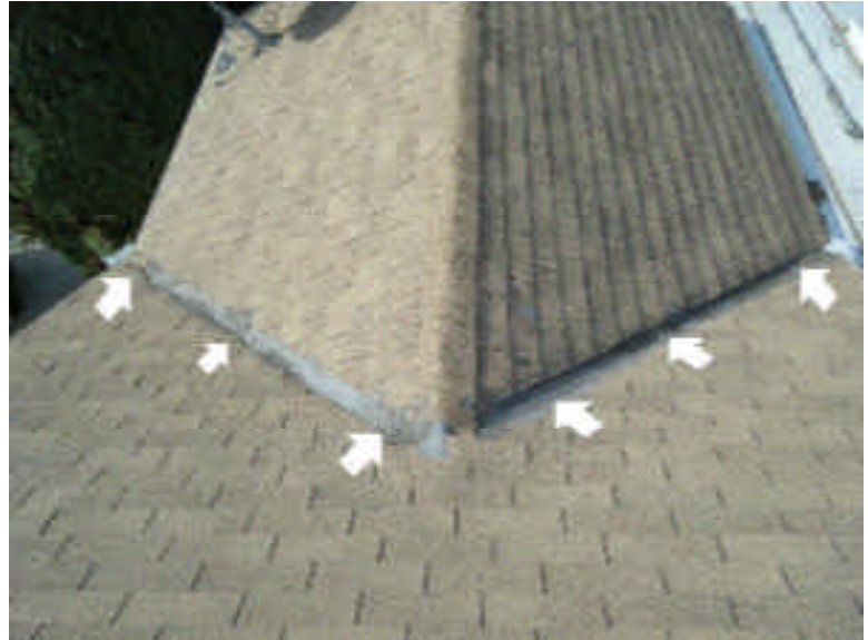
Needs Attention: On the composition roof , there is excessive mastic used in the back left valley joint.
