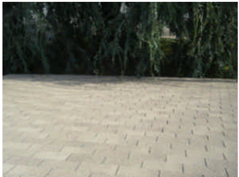
Needs Attention, there are tree branches growing over the roof and brushing against the structure which needs to be trimmed back.
