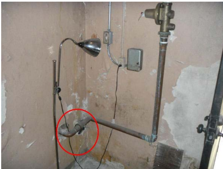
At the back of the building in the hall to the basement.
