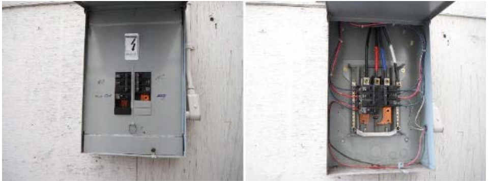
(exterior panel with missing breakers and exposed live components inside.
