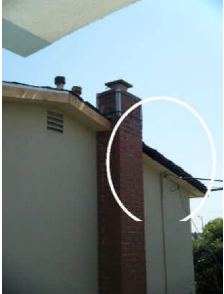
The back left edge along the roof is mid repair and the metal edge flashing is missing and the wood fascia piece.
