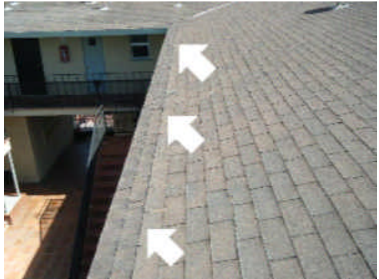
The front courtyard edges of the roof the roof appear to have been repaired recently.
