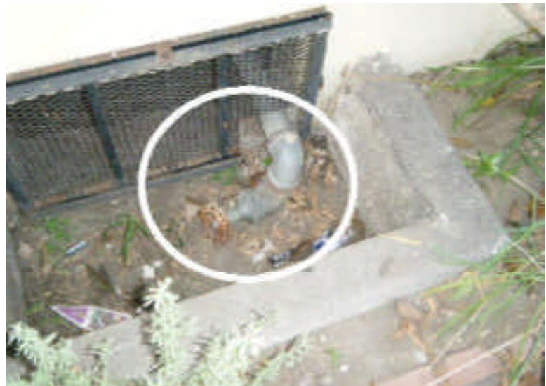
Crawl space access shut off
