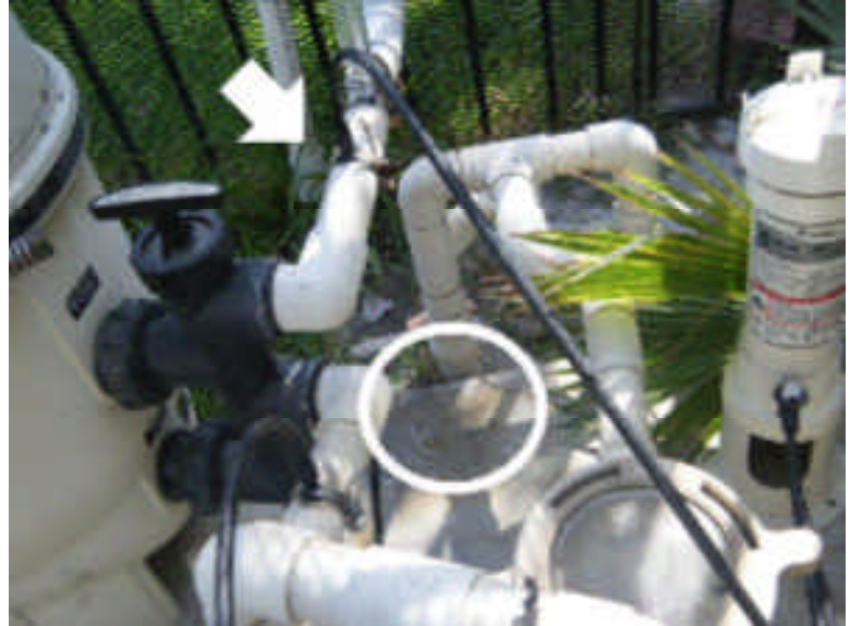
Needs Attention , there is a small leak by the filter.
