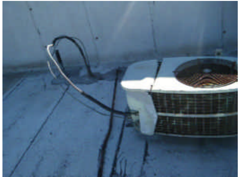
The condenser for the air conditioning is located on the roof.
