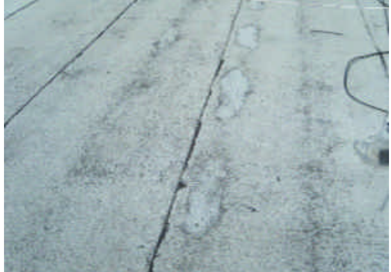
Close up view of worn area on left roof
