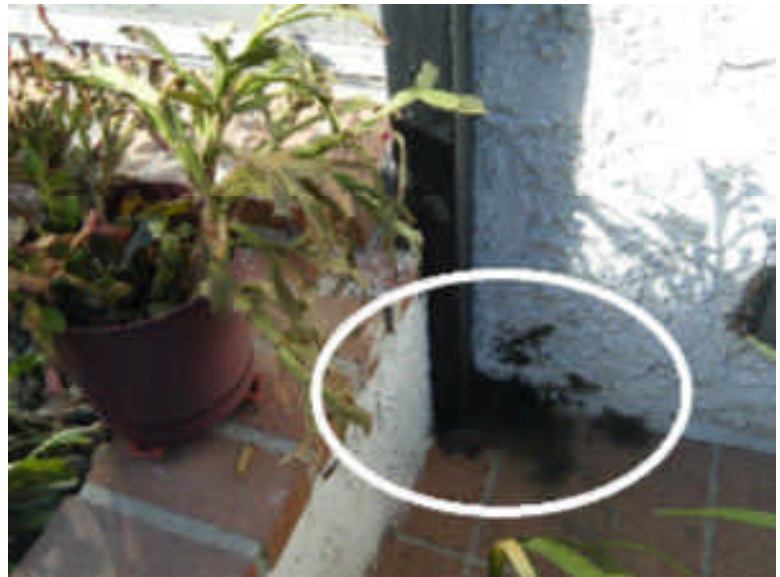
The tenant had put a vaseline on the joints in an attempt to seal this jointed area (the vaseline has aged and turned black)
