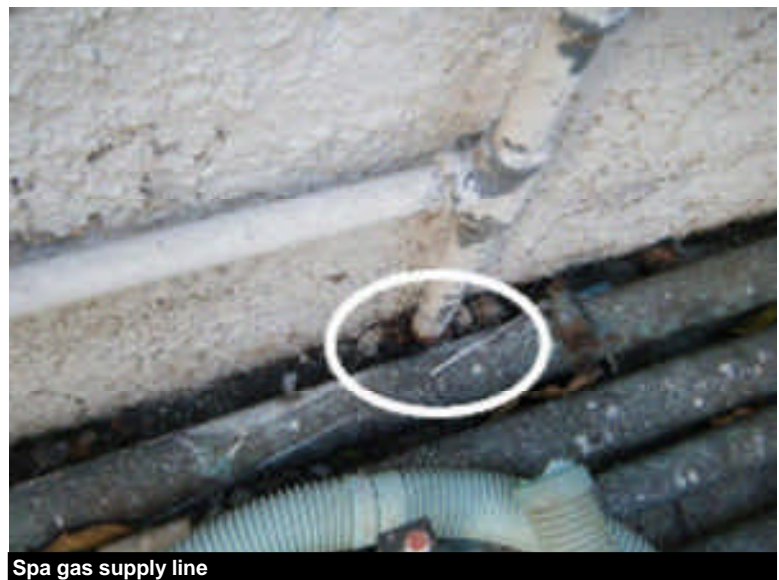
Spa gas supply line
