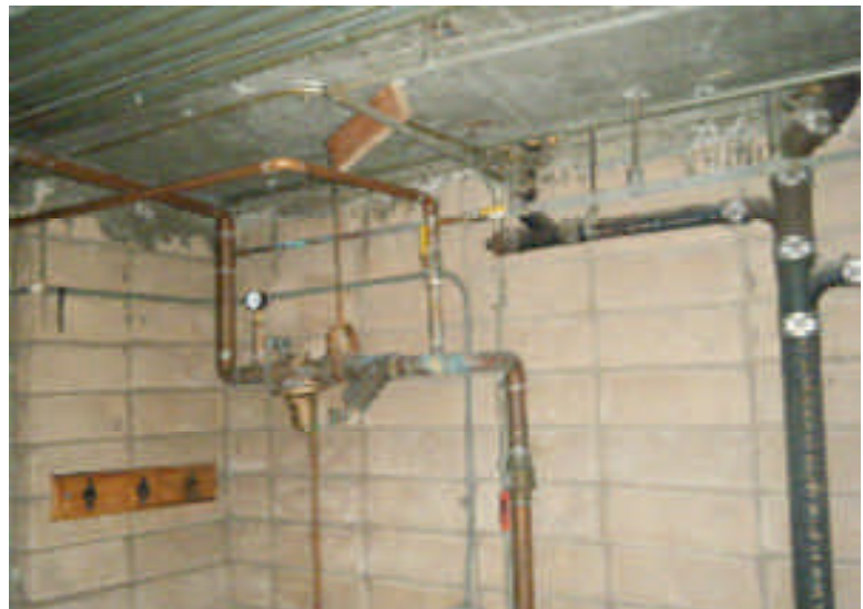
Left side water line and shut off
