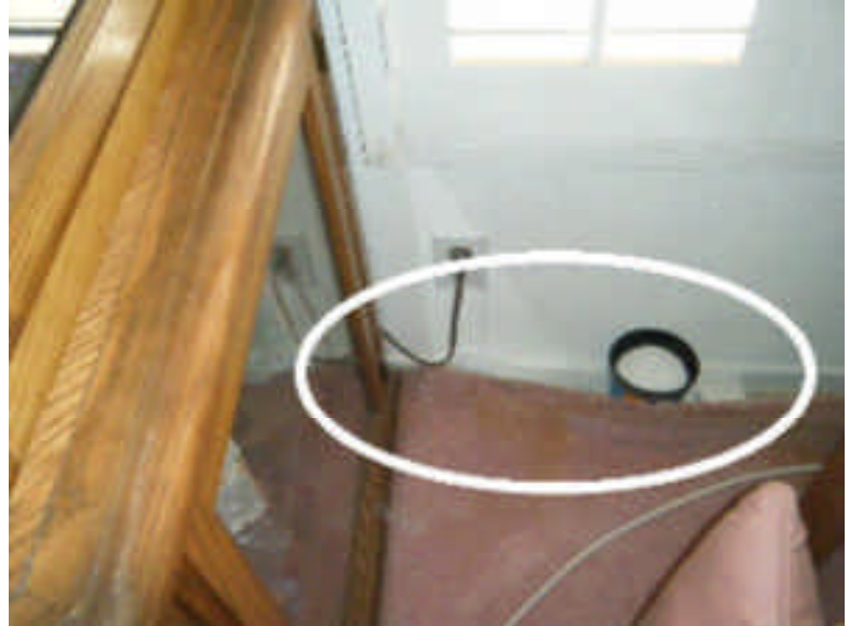
Not Acceptable. there are areas of moisture stains inside near the edge of the planter area.
