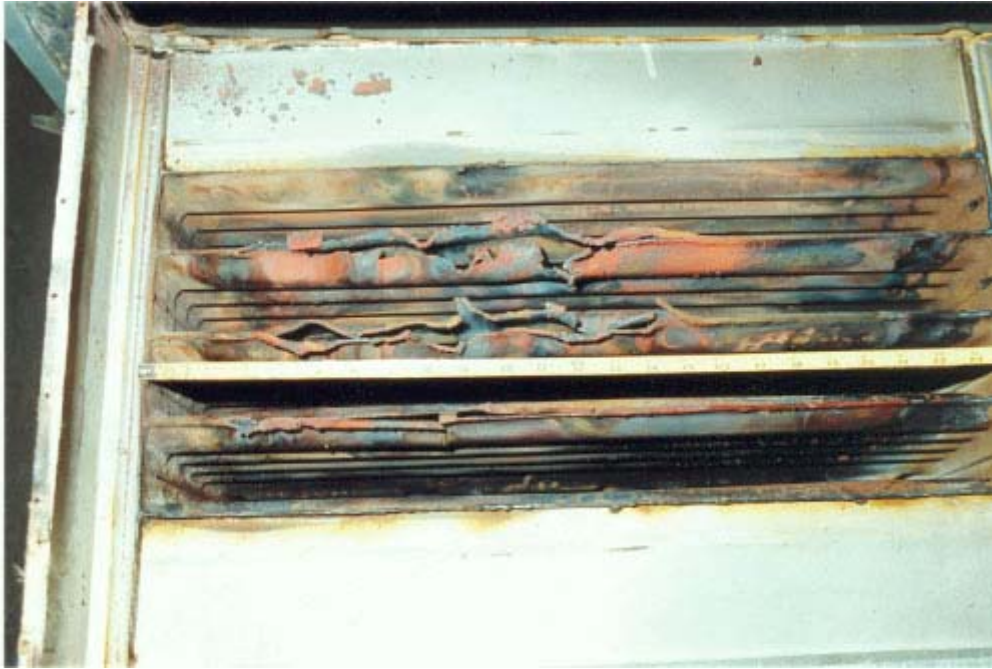
Photo Seven: Major failure of heat exchanger.
