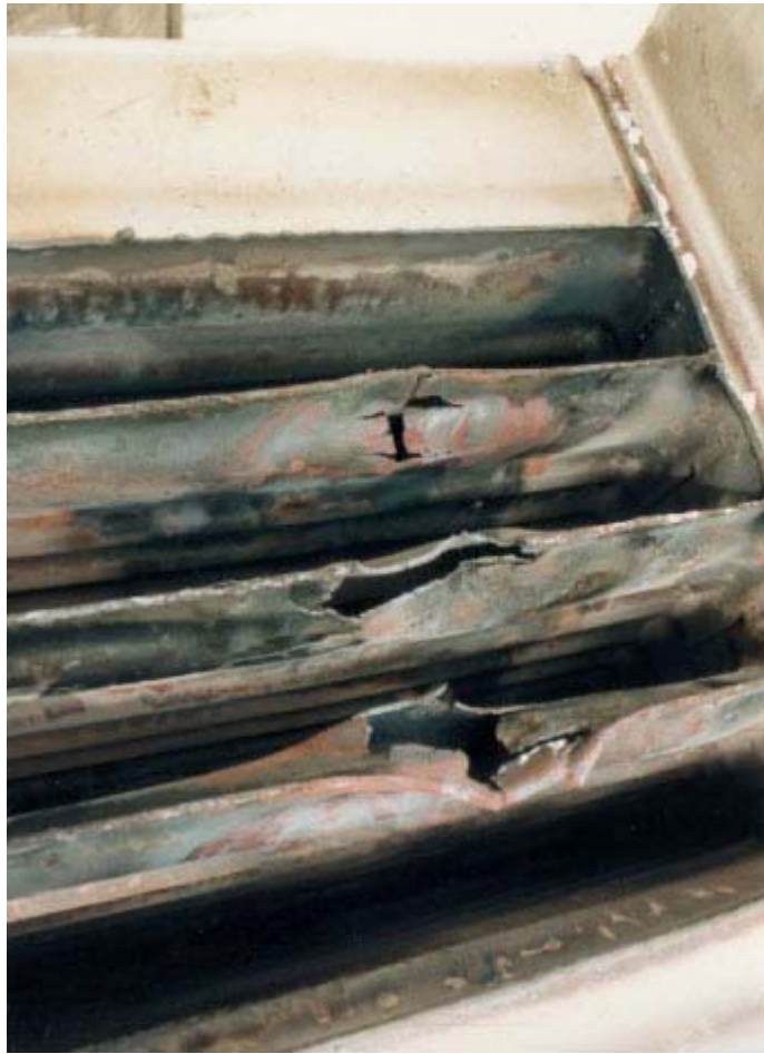
Photo Six: Failed heat exchanger.
